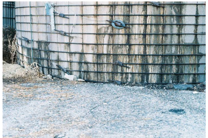
Base of silo showing deterioration of bottom row of staves. Photo used with permission of owner.
