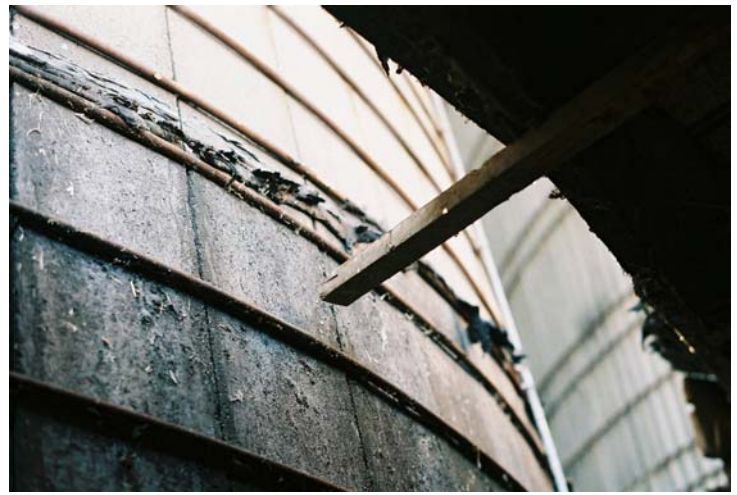
Silo (left) pulling away from the barn. The board in the center was used to monitor the rate of shifting. Photo used with permission of owner.
