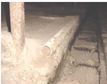
Photo 3: The Williams' simply lagged a 3 inch PVC pipe directly to the rear of the concrete stall base. Washers are sometimes used as spacers to provide drainage between the retainer and stall base.
